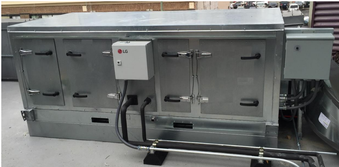
Figure 16. Rooftop Air Handler
